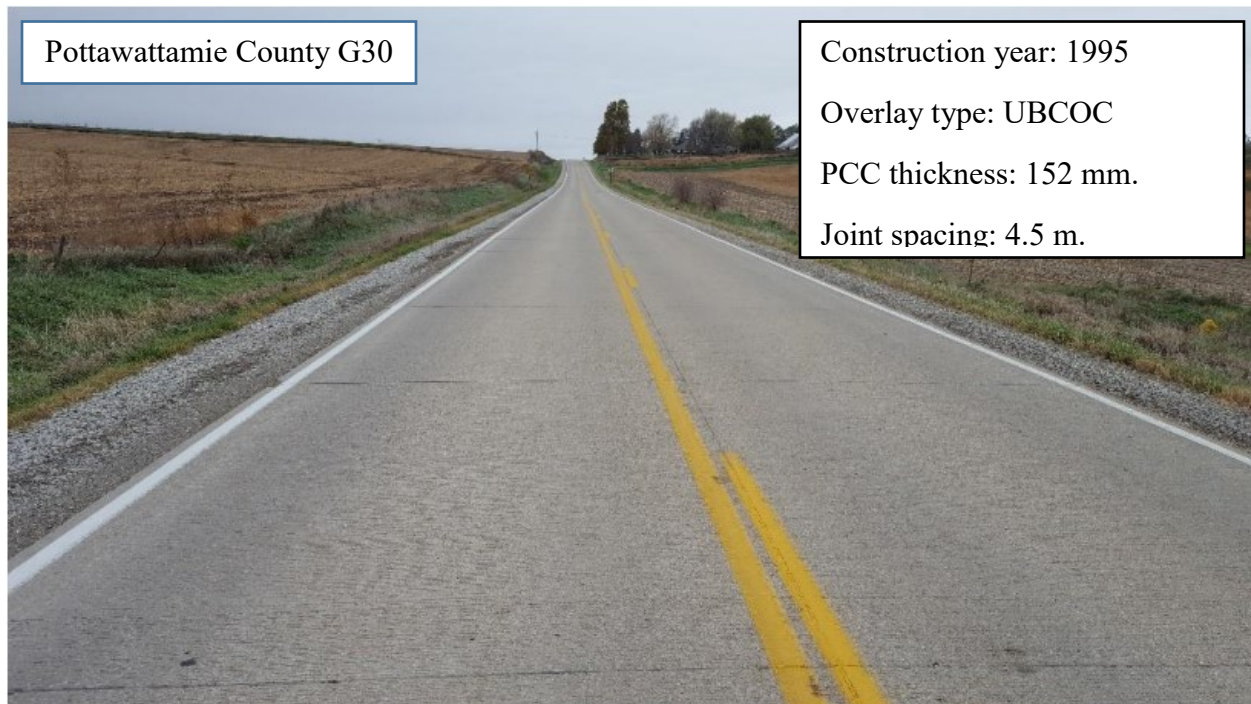
Figure 4-1 Surface condition on concrete overlay road in Pottawattamie County, Iowa
